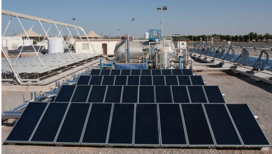
Fig.3.3.4. Flat plate solar thermal collectors. ( https://commons.wikimedia.org/wiki/File:MT-Power_Masdar_City.jpg , 2021).
