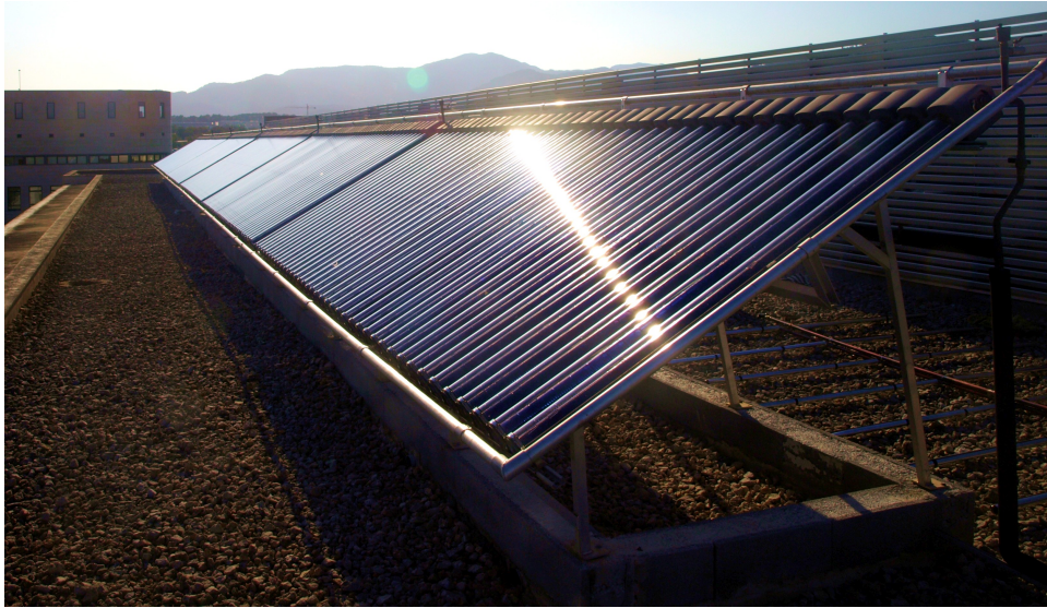
Fig.3.3.3. Solar vacuum tube collectors. (Source: https://commons.wikimedia.org/wiki/File:Col%C2%B7lectors_solars_de_tub_de_buit.JPG , 2021).
